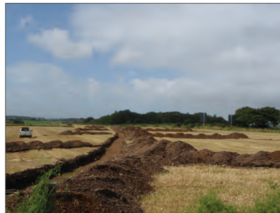
Plate 2: C5 - Evaluation trenches open taken from east, point where west end of bypass meets current A75.
